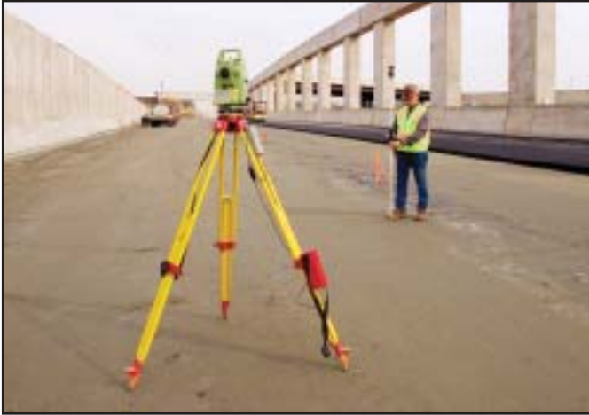
Archer Western used the Leica TPS1100 series in full robotic to bluetop the paving surface for I-285.
