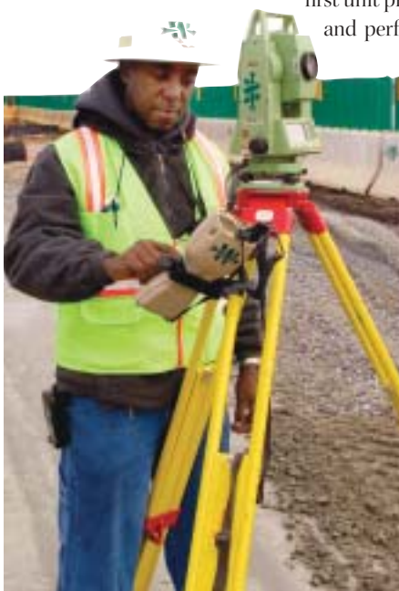
A surveyor on the Atlanta bridge project checks data in reflectorless mode.
